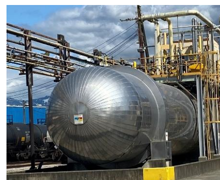
Above: one of three onsite chlorine storage tanks. Note that only one is used to store liquid chlorine, the other two have been converted to vacuum storage capable of capturing and storing all chlorine on site
