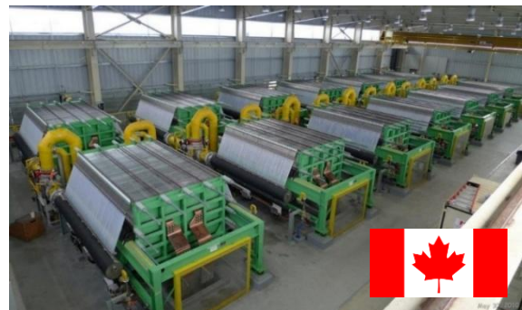
Above: Salt + Water + Electricity = Chlorine, a look at our cellhouse in North Vancouver
